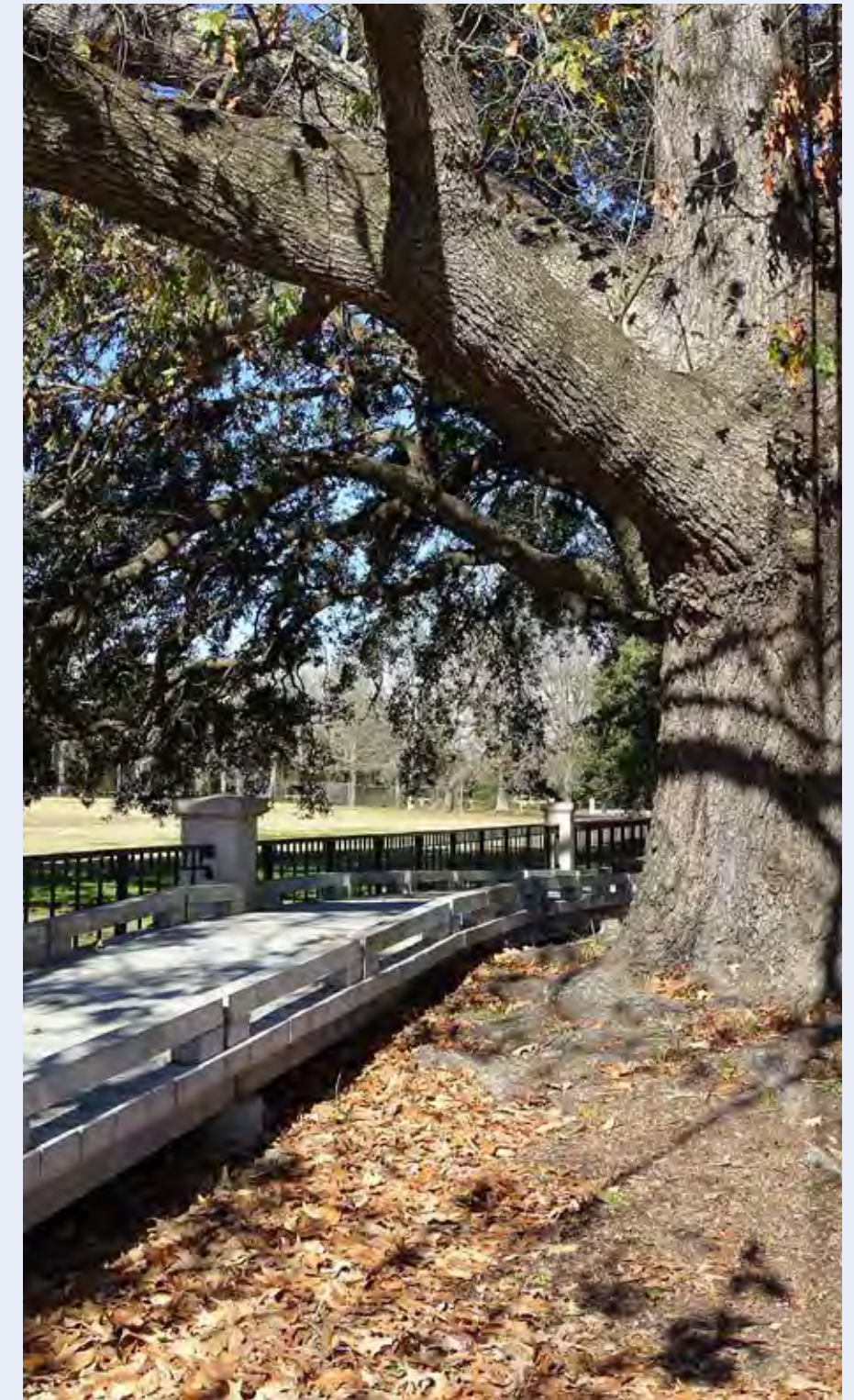
This tree along a Charleston park got help with root conflicts as the city built a bridge over the tree's roots.
